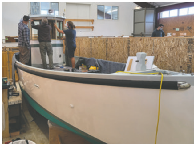
Team Clean Bay discusses conductor routing for AIS and VHF antenna wires.
